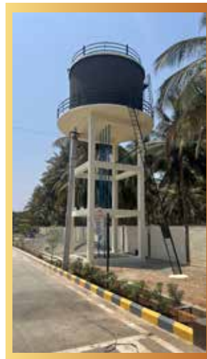
OVER HAED WATER TANK
